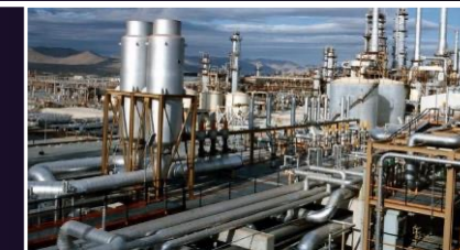
Real life Petrochemical plant
